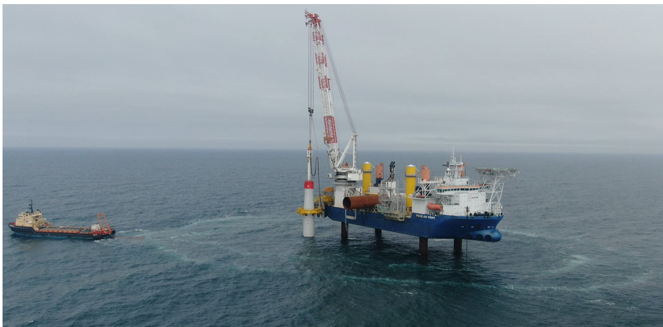
Figure 5. Air bubble curtain, seen as rings around the pile driving platform, during foundation installation for the Coastal Virginia OSW pilot project. Photo from Dominion Energy.
