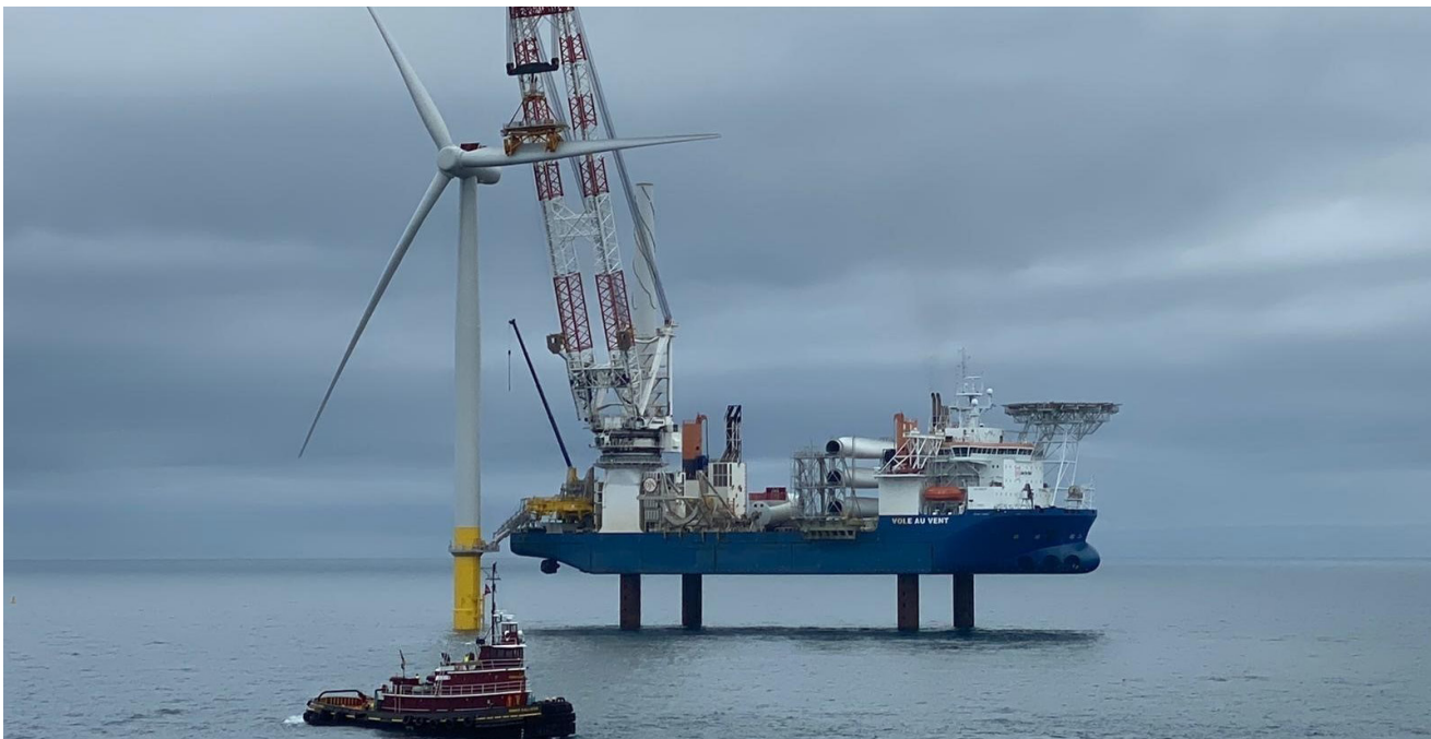
Figure 2. Jack-up vessel used for turbine installation at the Coastal Virginia Offshore Wind project. Photo by Dominion Energy .
