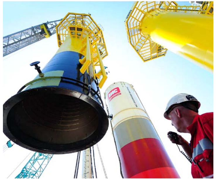
2013 start-up: the last of 30 monopile foundations was installed at EWE's 108MW Riffgat wind farm in September
