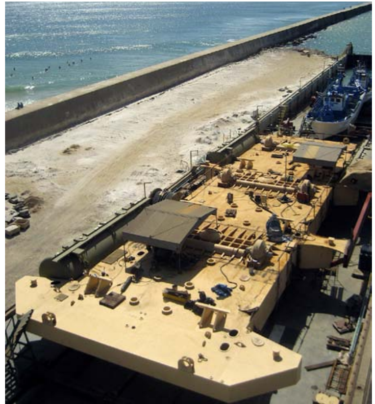
Behind schedule: three hinges are being attached to the WaveRoller vessel in Peniche shipyard
