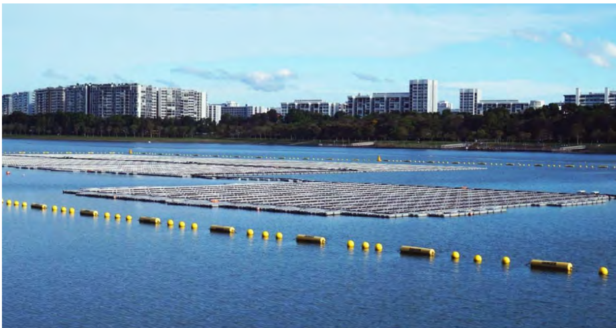
Floating Solar System in Reservoir
