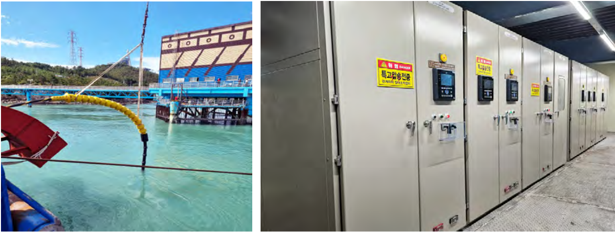
A picture of the submarine cable laying and offshore substation facilities (Courtesy: KIOST)
