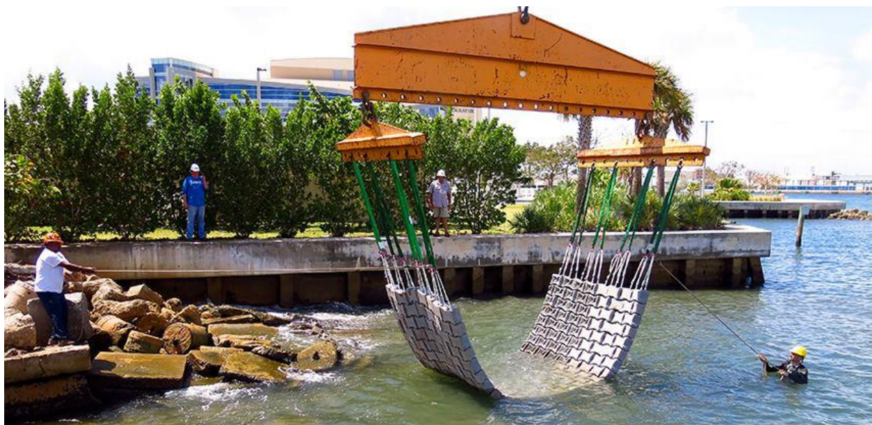
(Fig. 5) Deployment of one of the ECONcrete® Bio-Enhanced Marine Mattresses used for this study.
