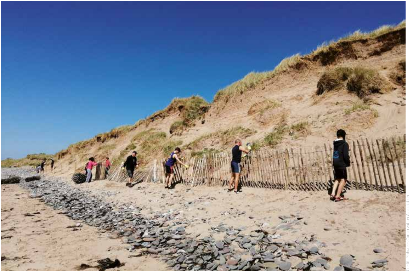
Figure 5.1 Example of community-led Nature-based Solution (installation of dune fences) to mitigate wind-blown sand leading to closure of the road in the Maharees Peninsula, Ireland.
