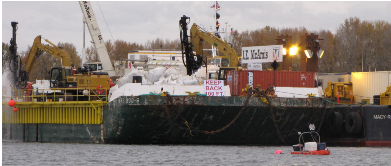
Figure 4.4. A View of the Barge in Line with the Drilling of the Holes for Blasting
