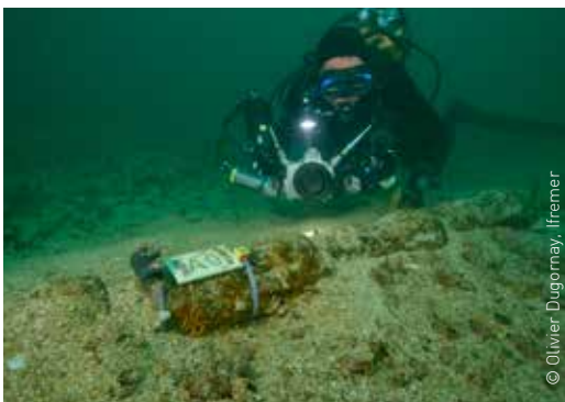
Fig. 53. In situ monitoring of the Paimpol-Bréhat cable.
