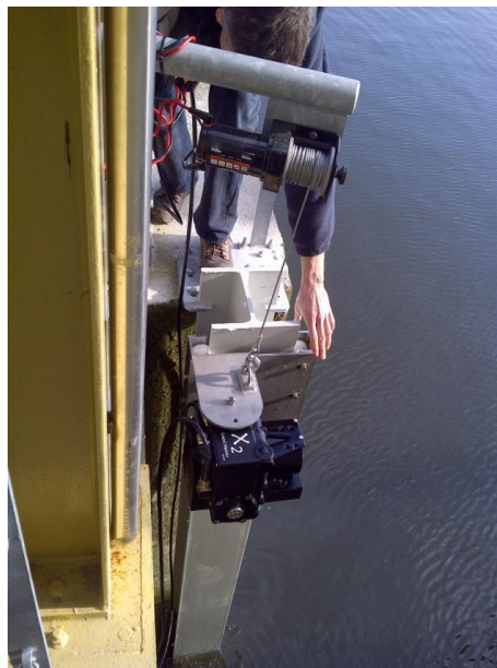
Figure 8.3 Mounting at Arzal dam, France
