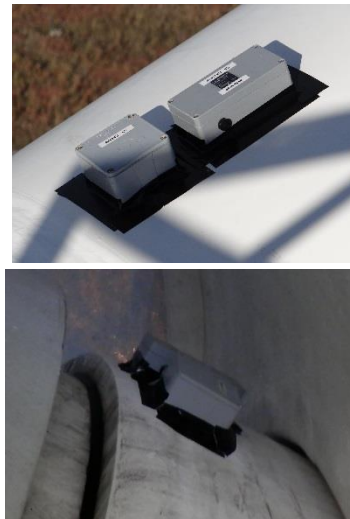
Figure 2.1.3. Placement of the vibration sensors – (top) external or (bottom) inside of the shroud over the hub.
