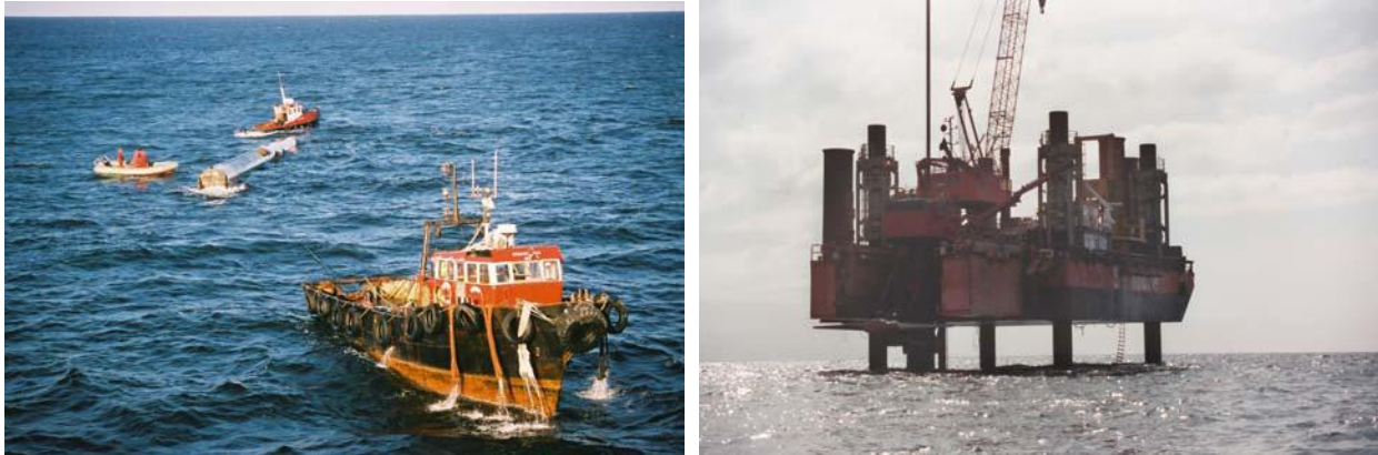
Figure 4 : Installation of the monopile for the "Seaflow" marine current turbine off Foreland Point near Lynmouth (Photographs from MCT Ltd)
