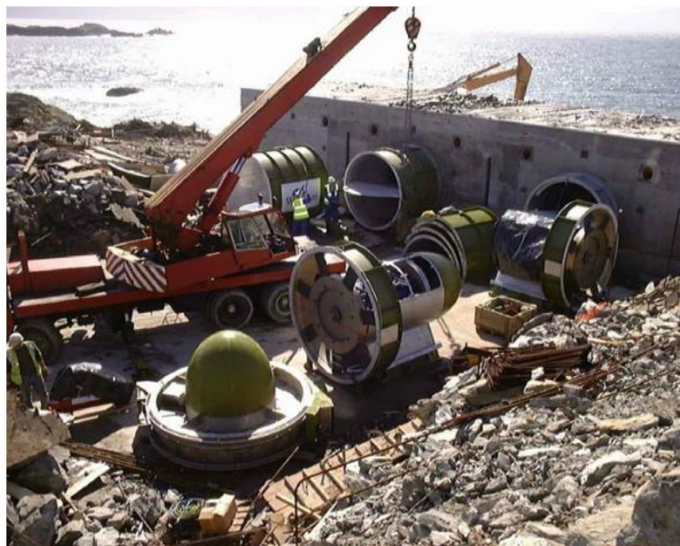
Figure 4.3 Turbine and duct valves of the LIMPET plant
