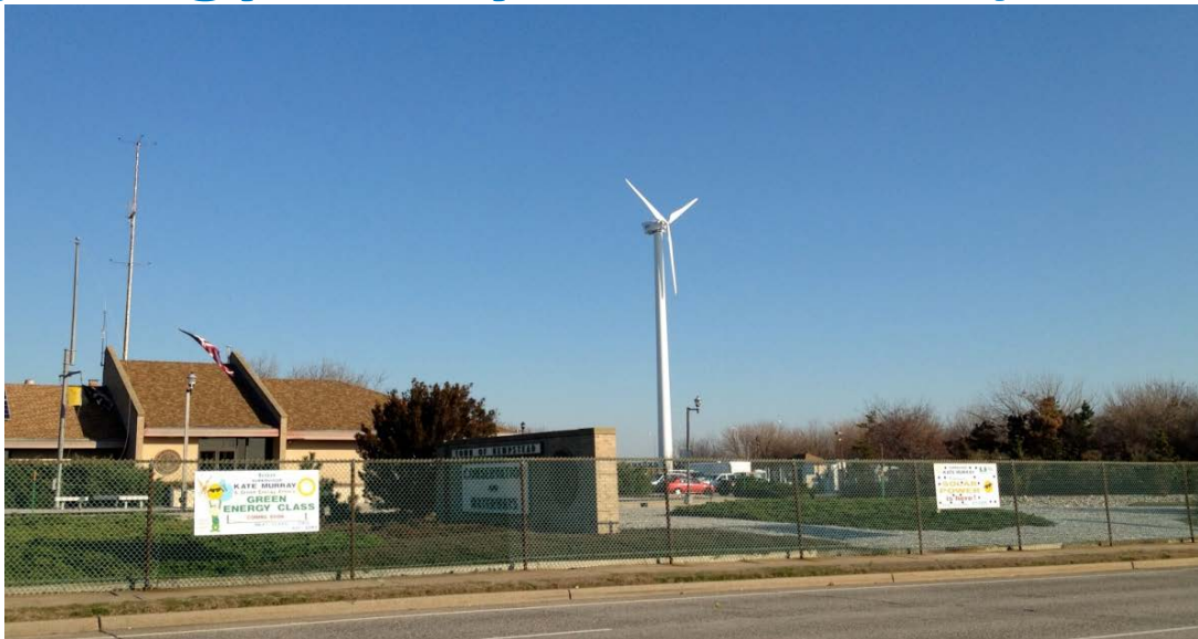
Northwind 100, 100-kW wind turbine; Hempstead, New York. Photo by Town of Hempstead, NREL 28963
