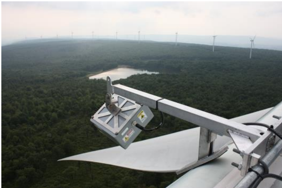
Figure 2. Photograph of the Deaton UAD secured to the wind turbine by a cantilevered arm.
