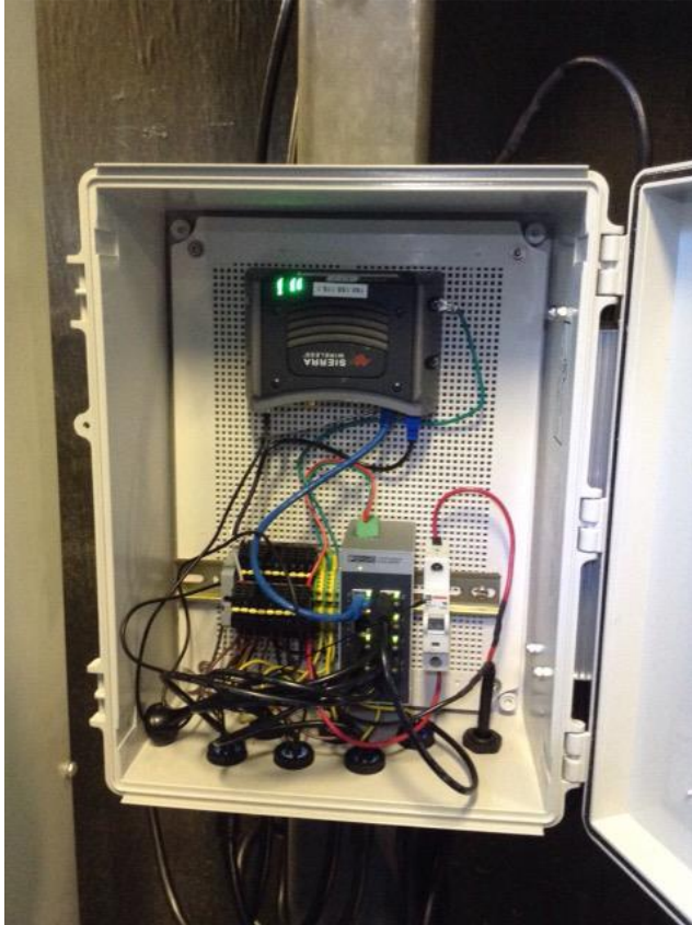
Figure 5. The communications box for the ultrasonic acoustic deterrent system.
