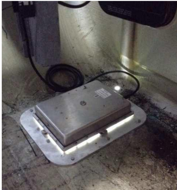
Figure 9. Photograph of a prototype UAD installed on the floor of the nacelle.
