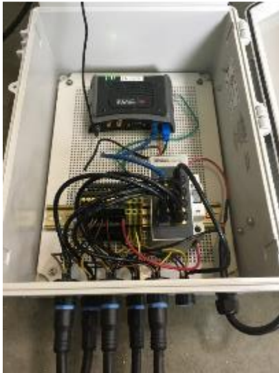
Figure 20. Photograph of the power supply box, modem, Ethernet switch and circuit breaker.
