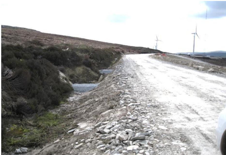
Regular, robust check dams on road sloping ditches
