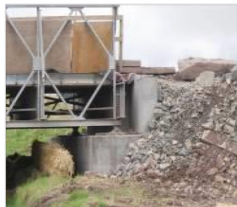
Bridge and bank habitat. Steep sides of loose material could be washed off in a storm event. Use of splash boards on bridges can prevent contamination of watercourses.
