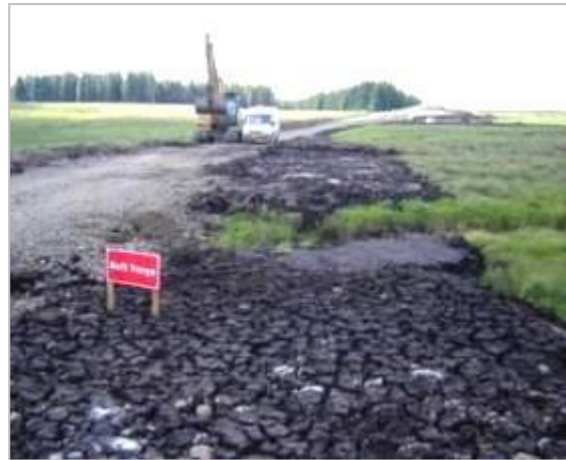
An example of bad practice. Excavated peat placed 4m from edge of access track. Note that no peat turves have been re-used. This peat is likely to dry out and provides no ecological benefit.
