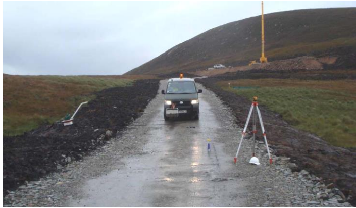
Surveying floating road structural integrity. Note that excessive material should not be placed on the side of tracks as shown on the left of this image.
