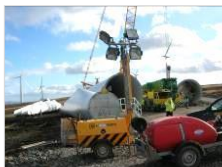
Considerable lay-down areas are required on site and should be planned for early in the process.
