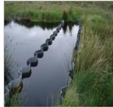
Blocked drainage ditch using plastic sheet dam
