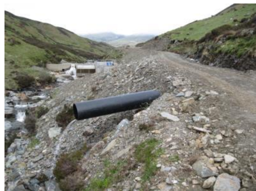
Culvert under road – better attention to detail would 'hide' the exposed pipe.
