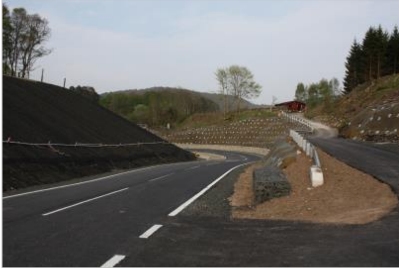
An example of the scale of improvements which can be required on the public road network
