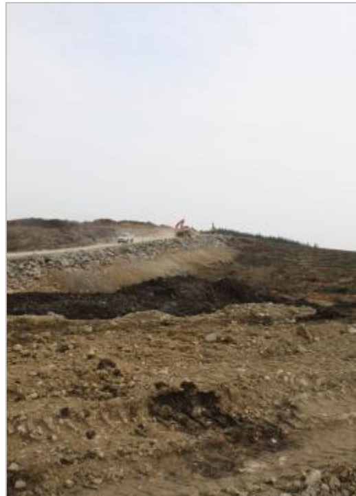
A very steep track edge which should be properly restored post construction.
