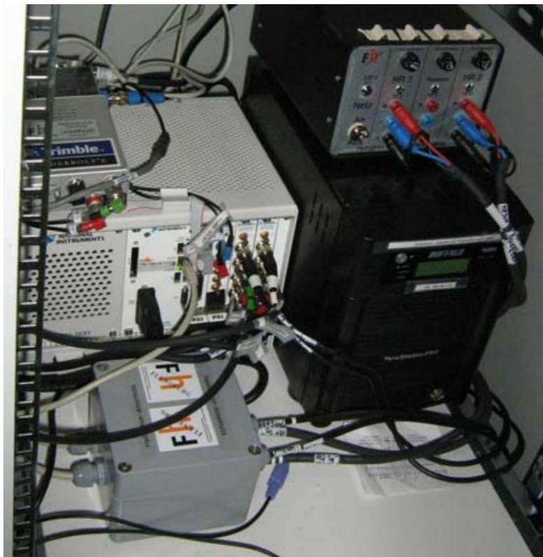
Fig. 6.1.3: Measuring computer and measuring equipment on AV04 (Photo: BSH)
