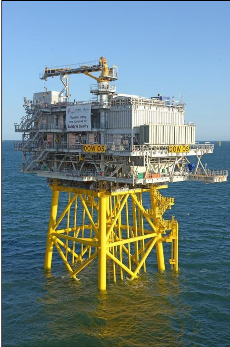
Figure 3.3-5 Example of an Offshore Substation on a Jacket Foundation (Equinor-operated Dudgeon Offshore Wind Farm)
