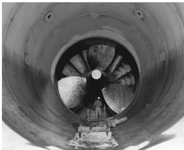
Fig. 9. Propeller turbine of the Shihwa tidal power plant (Seo, 2010).
