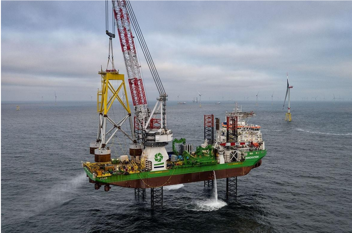
Figure 2.5 Installation of a suction bucket jacket at 'Borkum Riffgrund 2' in 2018 (copyright Örstedt/Matthias Ibeler, source: https://orsted.de/presse-media/news/2018/07/bkr02-letztes-sbj-installiert 06.12.2018).
