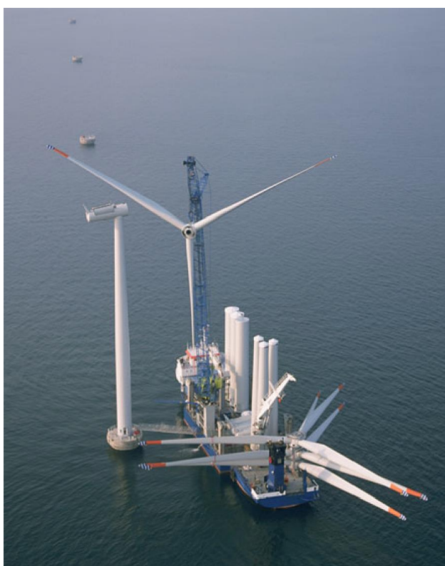
Figure 2.11 An assembled rotor being lifted onto a nacelle at Nysted windfarm (©DONG Energy)
