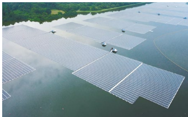
60 MW Floating Solar in Tengeh Reservoir
