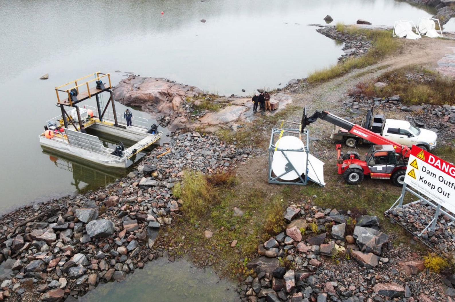
One of the five-Waterotor turbines manufactured this summer and installed at the CHTTC. A 3-turbine array will be operating coming winter at the CHTTC.
