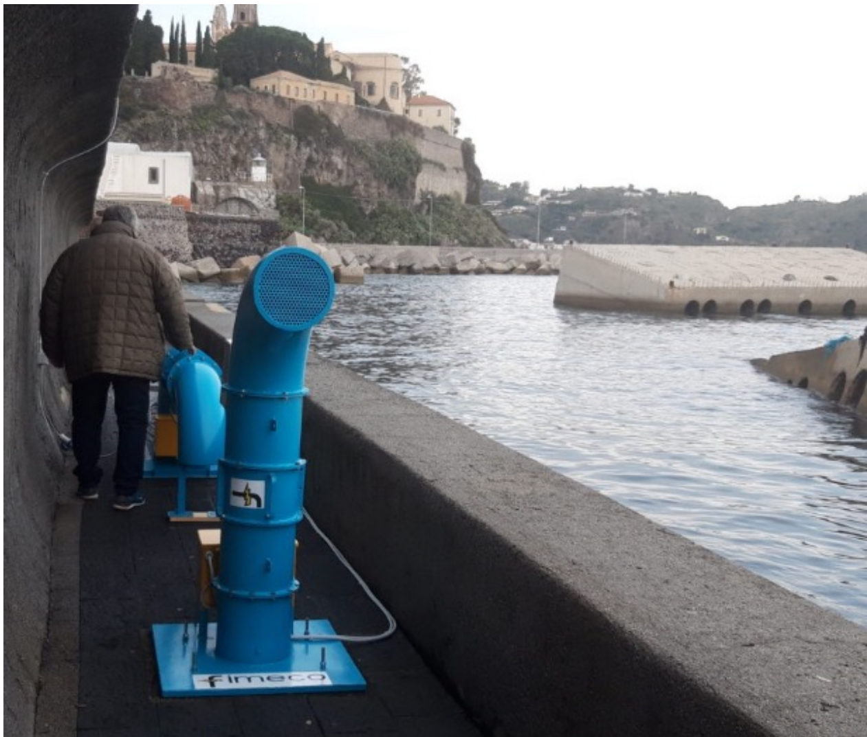
The turbine developed by Fimeco and Enermedsea installed in Lipari island breakwater barrier
