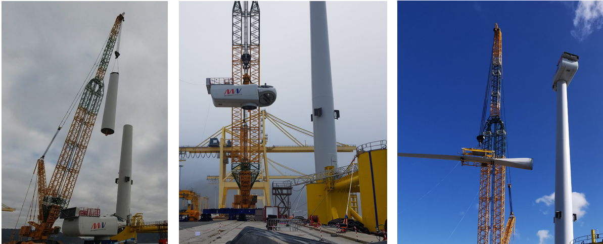
Figure 9. Integration of wind turbine components with a crane (tower [left], nacelle [middle], and blade [right]). Photograph of the WindFloat Atlantic project courtesy of Principle Power and Ocean Winds.
