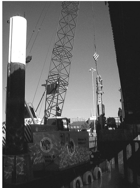
(b). The impact driver being held on the top of a pile for driving purposes.
