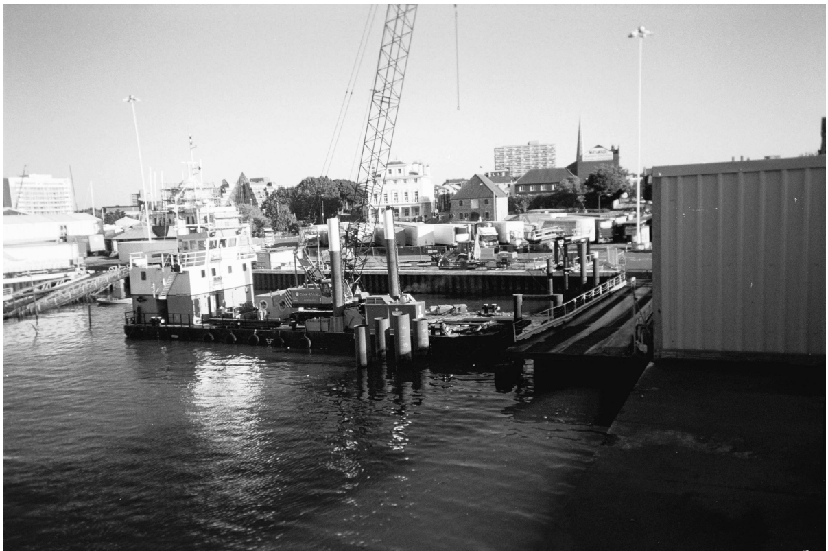
Fig. 9. Photograph of site during piling operations. The two groups of four piles to one side of the linkspan can be seen. The other two piles (numbers 9 and 10) are obscured by the structure (pedestrian walkway) on the right of the photograph. One pile in each of the groups was left standing proud, for later dynamic testing purposes using the impact driver.
