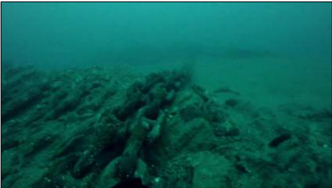
Figure 42. Section of the lower catenary corresponding to mooring leg 5 settled on outcrops.
