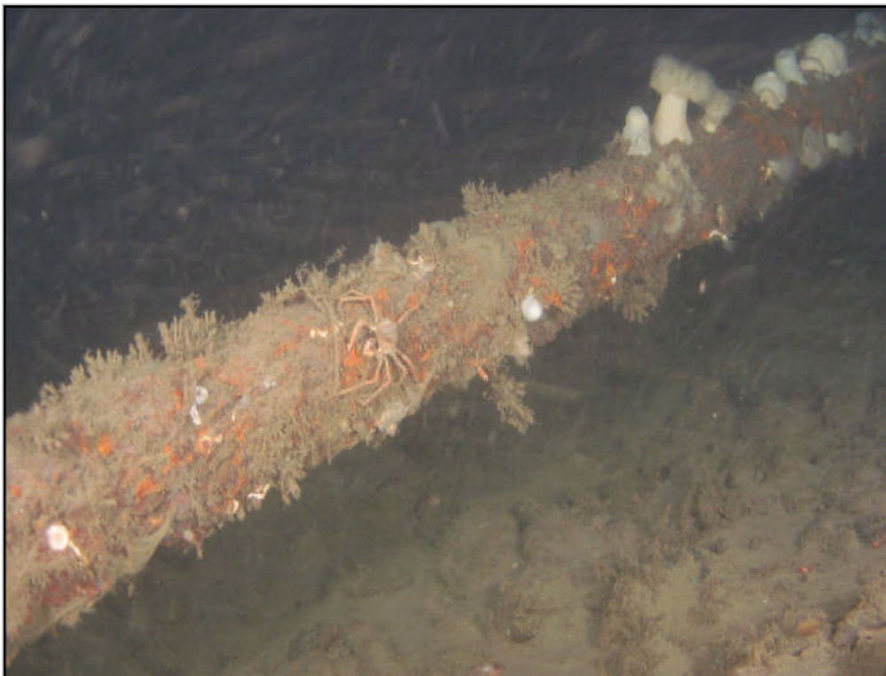
Fig. 50 Subsea power cable, in place for approximately 50 years, covered with sessile encrusting organisms at Vancouver Island (BCTC 2006).
