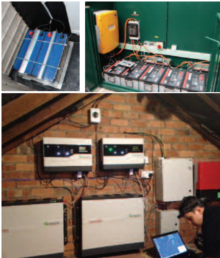
Figure 2.31 Lead acid and Lithium Ion batteries used in the SOLCER retrofits.
