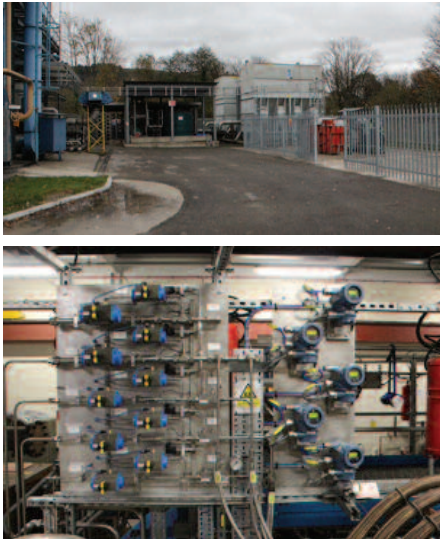
Figure 5.2 The 5-Gas Mixing facility with gas storage hard standing.
