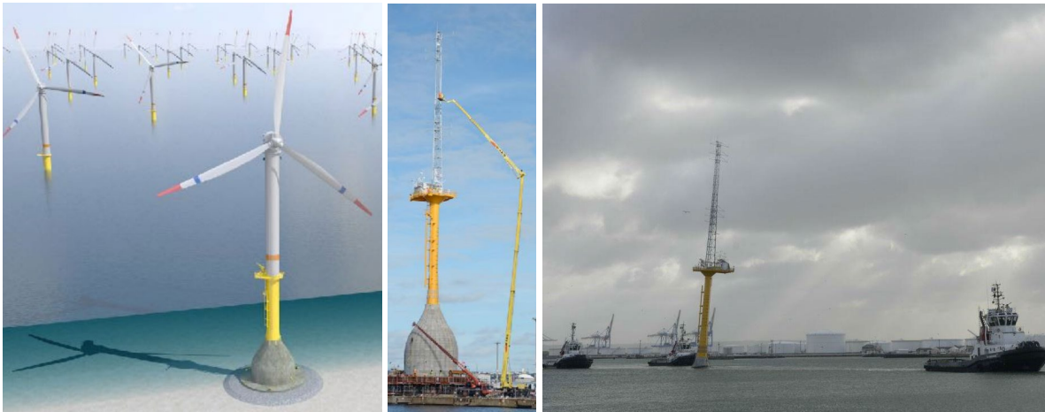
Fig. 12. Cranefree gravity base foundations: concept for an OWF using gravity base foundations (left). Construction of a foundation with a metmast in Fécamp, France (middle). Towing the metmast and its foundation to sea (right). © Seatower A/S.
