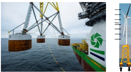
Fig. 13. Installation of a suction bucket jacket (left, OWF Borkum Riffgrund 2, © Ørsted). Idealised SBJ loading (right, OWF Borkum Riffgrund 1, Ørsted (2019)).
