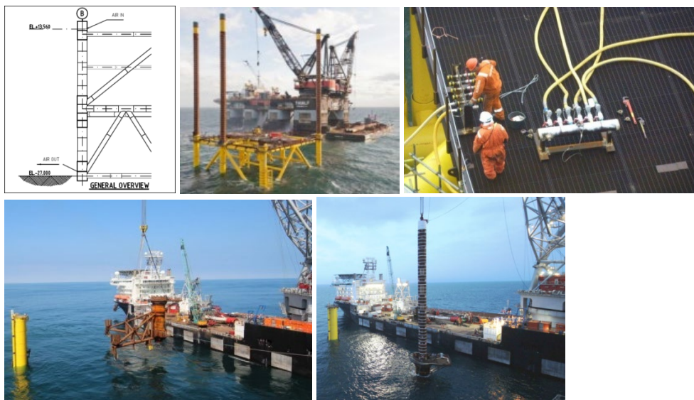
Fig. 5. Schematic drawing (top left) and application of jacket legs extending above the water surface and thus acting as cofferdams at Dolwin alpha (top middle); air hoses for dewatering the pile sleeve (top right) at DolWin alpha; Installation of a cofferdam extension on top of the pile sleeve (bottom left) and piling through the complete cofferdam at BorWin beta (bottom right) © TenneT
