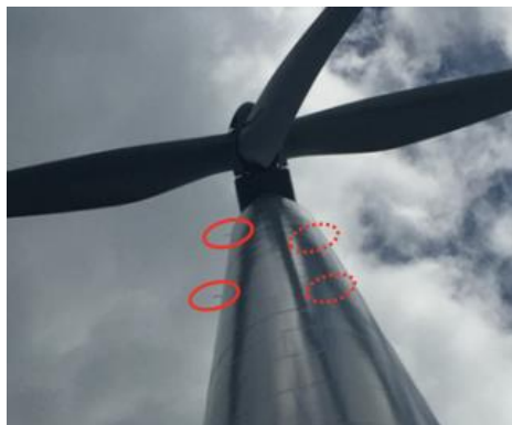
Figure 2. Photo of installed nozzle on tower section platform from outside of wind turbine
