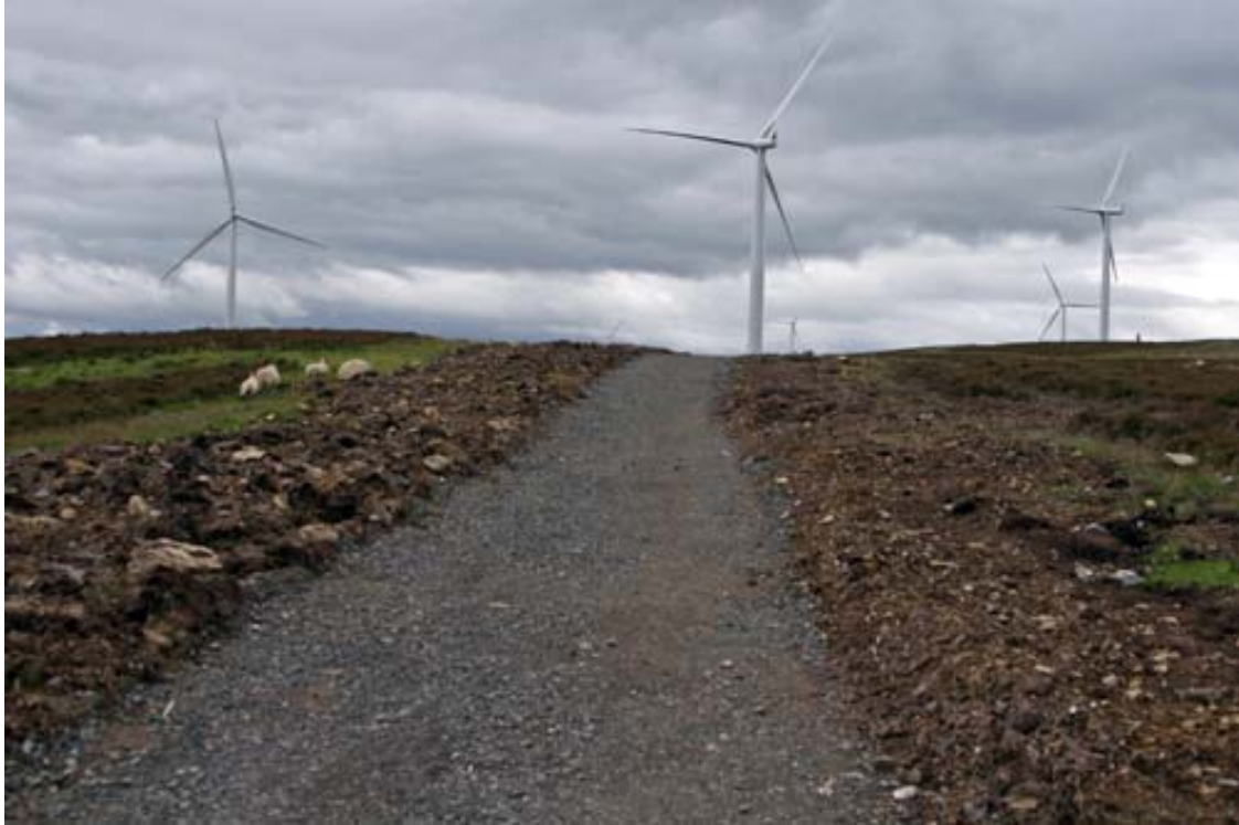
Wind turbine road showing 5 meter wide area of disturbance and habitat damage
