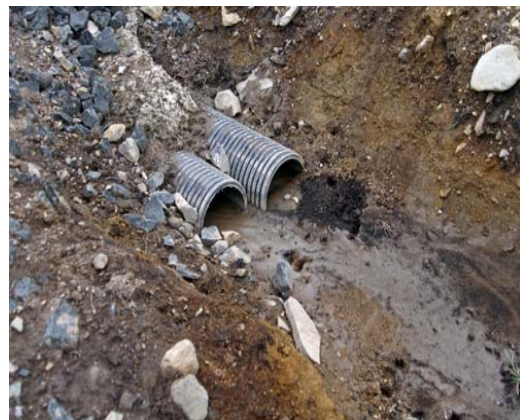
Erosion and siltation problems on site
