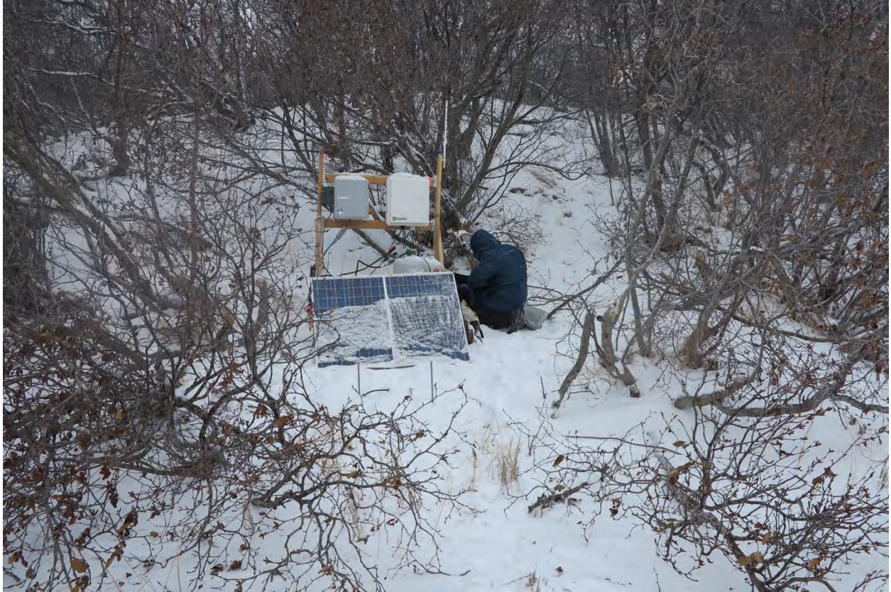
Figure 38. UAF personnel working on the remote power/real-time data telemetry system in February, 2017.
