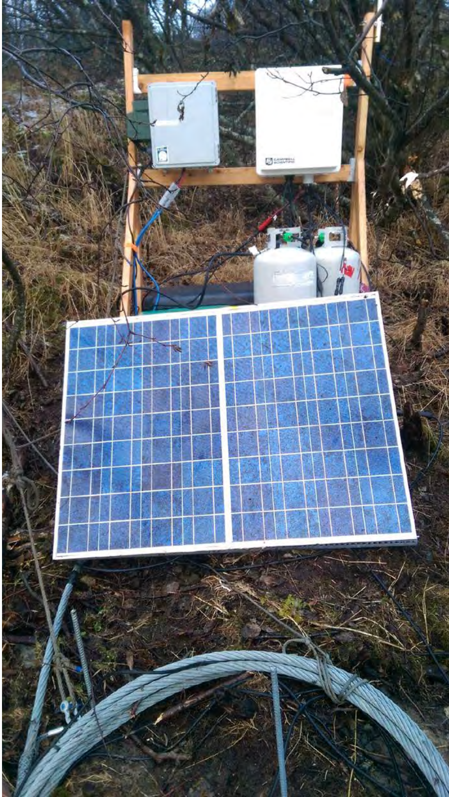
Figure 33. Power System with Solar Panels, November, 2016.
