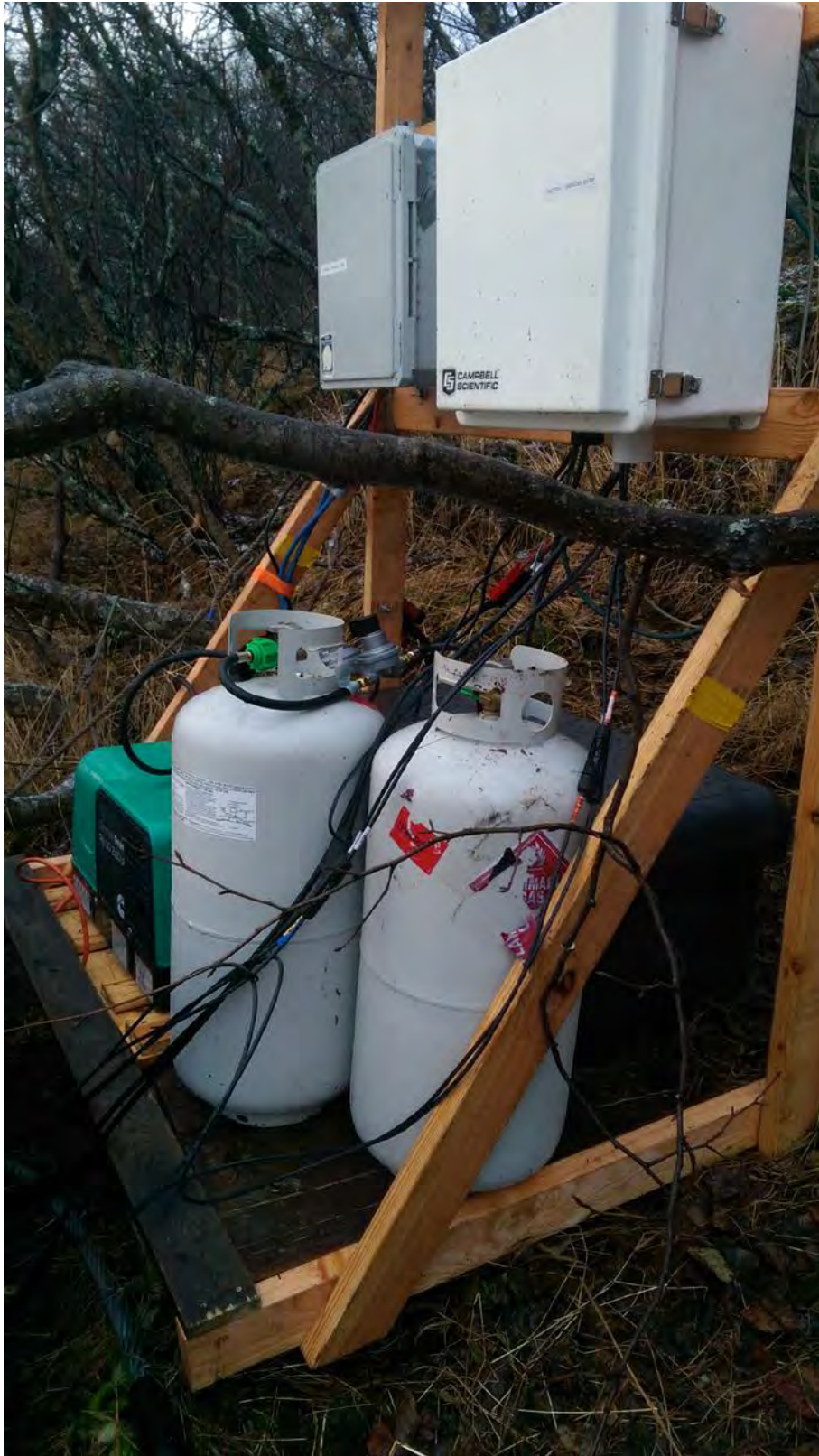
Figure 34. Remote power and data telemetry system, November, 2016.
