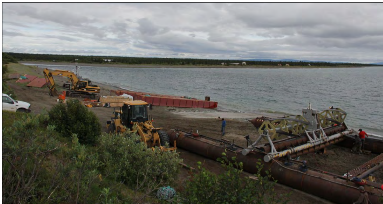
Figure A-5. RivGen staging on Lake Iliamna, July 2015.
