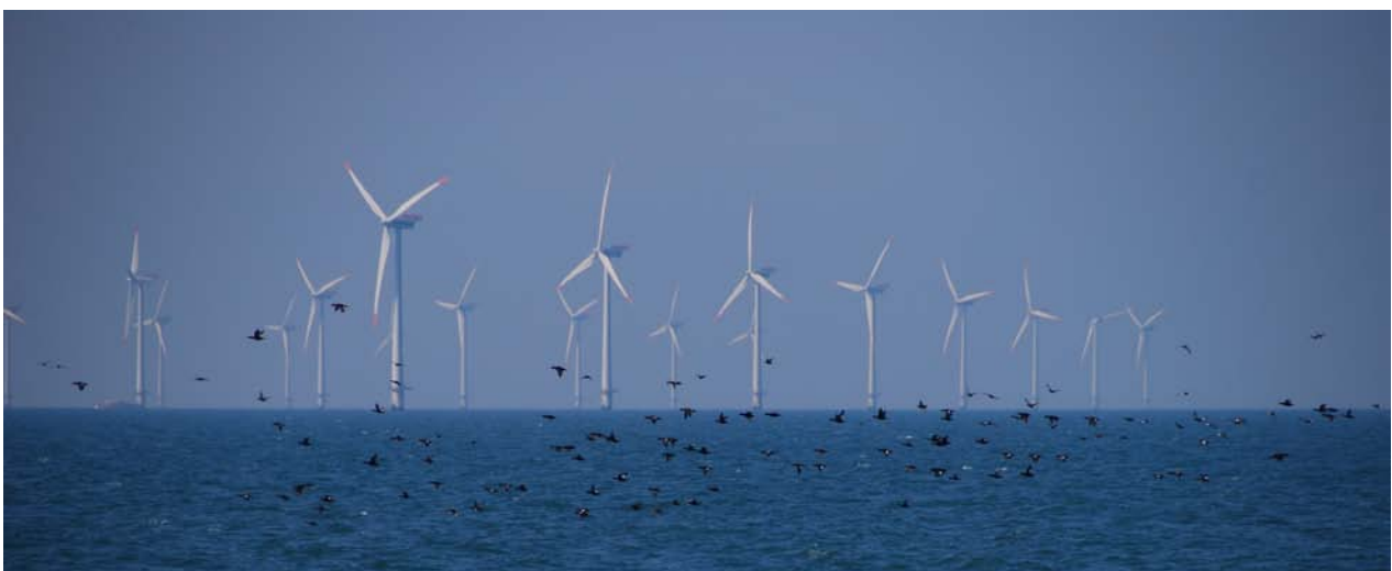
Horns Rev 1 Offshore Wind Farm
