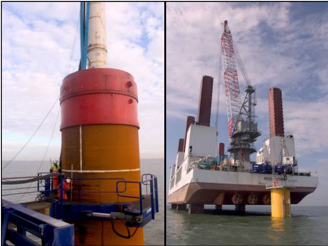
Plate 2.3 Monopile foundations being installed at Kentish Flats by the jack up vessel Resolution
