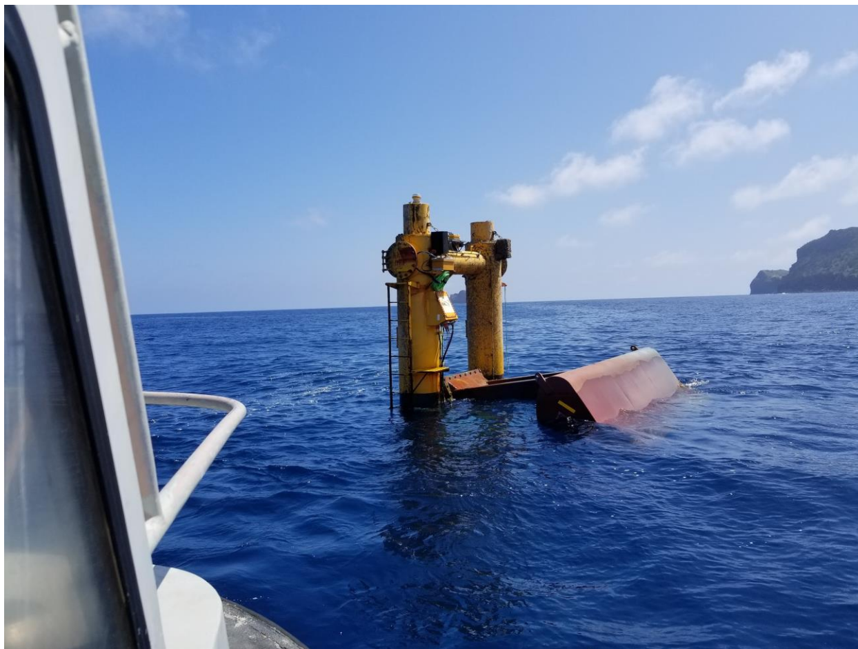
Figure 1.10. Advanced Azura Prototype during an inspection by Sea Engineering at WETS in spring 2018. Note larger float with greater moment arm, as compared with baseline Azura.
