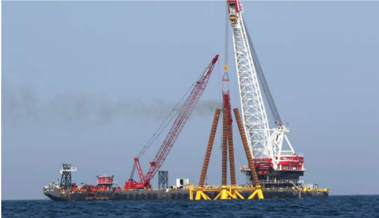
Figure B-5. 08/18/2015 Offshore Photo 0111: Weeks Barge 533 piling at WTG2 with diesel hammer (notice smoke).
