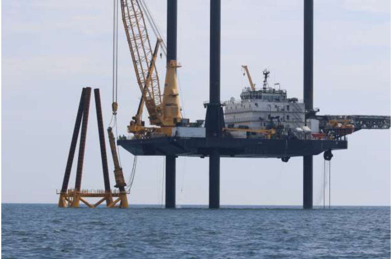
Figure B-17.9/17/2017 Offshore Photo 2352: Lift Boat Roberts driving the first pile at WTG 5.
