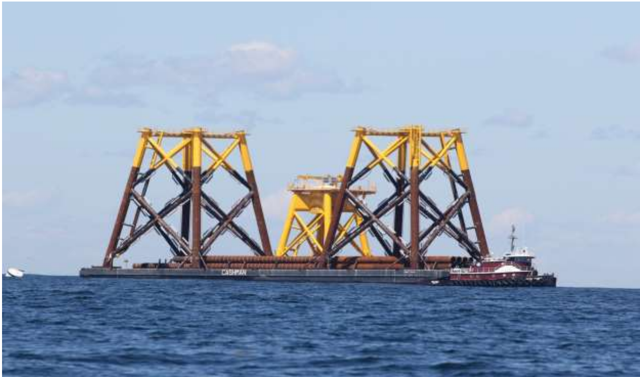
Figure B-8. 8/15/2015 Offshore Photo 0014: Two foundations, WTG 2 transition deck, and piles aboard the Cashman barge with support tug Reed Danos. Anchor buoy visible.
