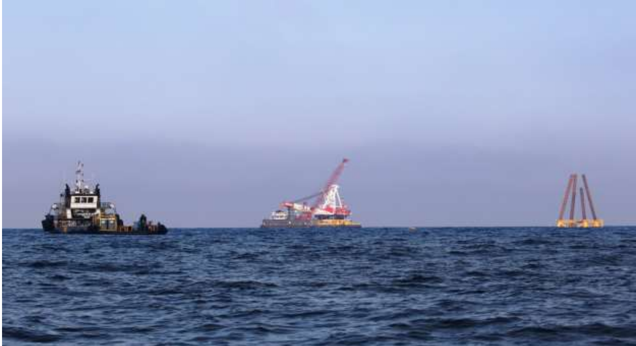
Figure B-11.8/26/2015 Offshore Photo 0581: Supply vessel Josephine Miller and Weeks derrick barge 526 at WTG 2. WTG 3 is to the far right with four piles ready to be driven.
