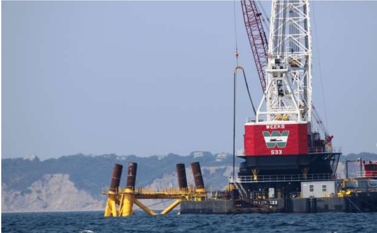
Figure B-15.9/02/2015 Offshore Photo 1010: WTG 3 with first set of piles driven by Weeks Derrick Barge 533. Block Island in the background.
