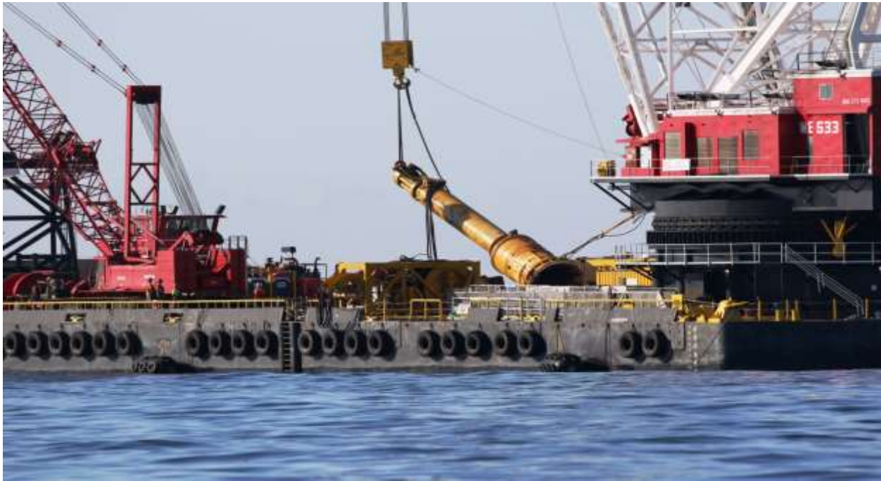
Figure B-12.8/29/2015 Offshore Photo 0622: Hydraulic hammer being lifted from Weeks Derrick Barge 533.
