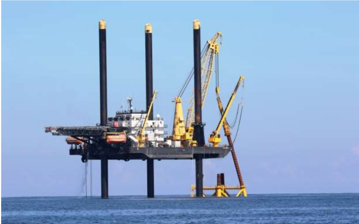
Figure B-16.9/19/2015 Offshore Photo 2542: Lift Boat Roberts driving the last pile at WTG 1.
