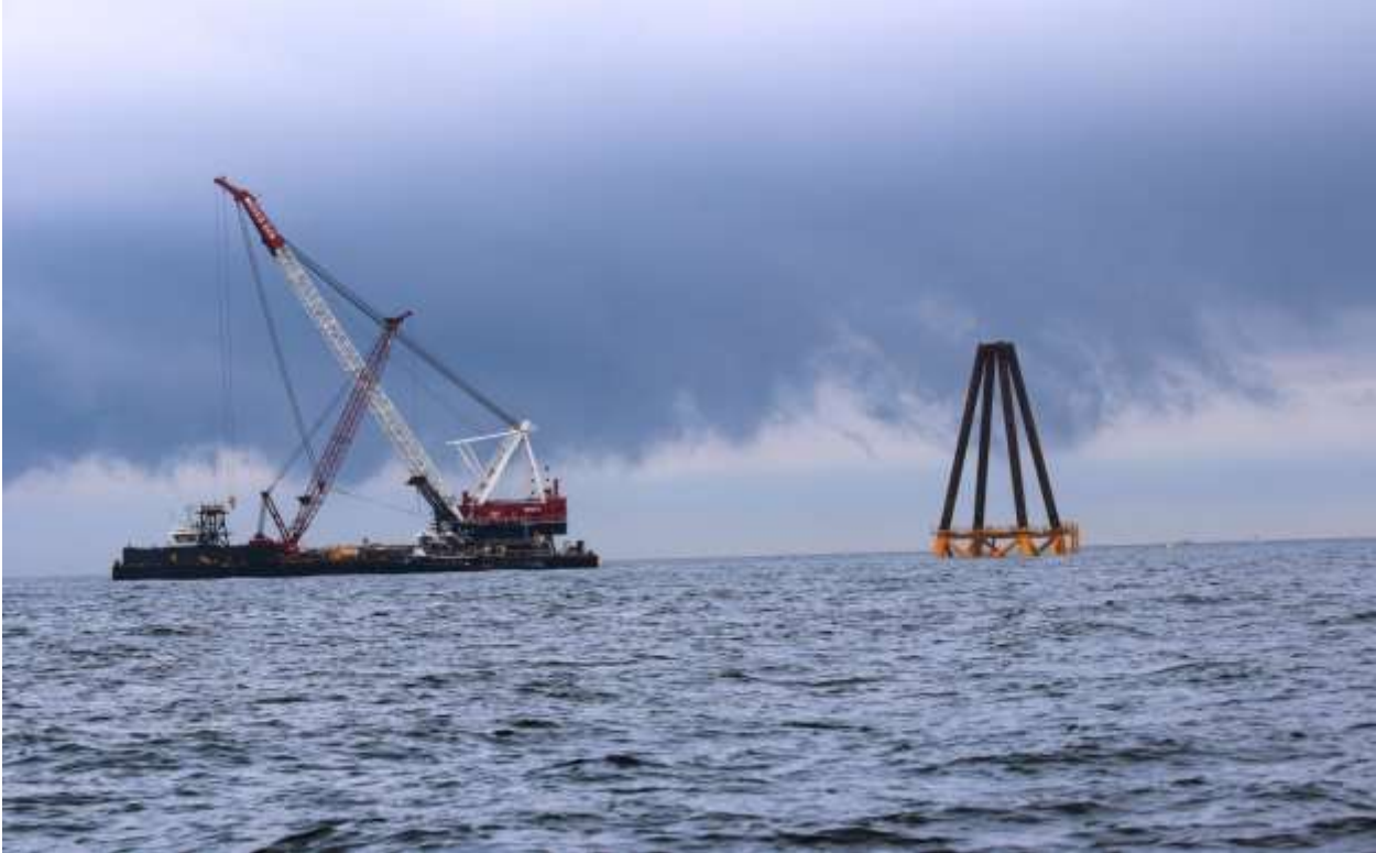
Figure B-21.9/20/2015 Offshore Photo 2579: Weeks Barge 526 next to WTG 5 with second set of piles in place.
