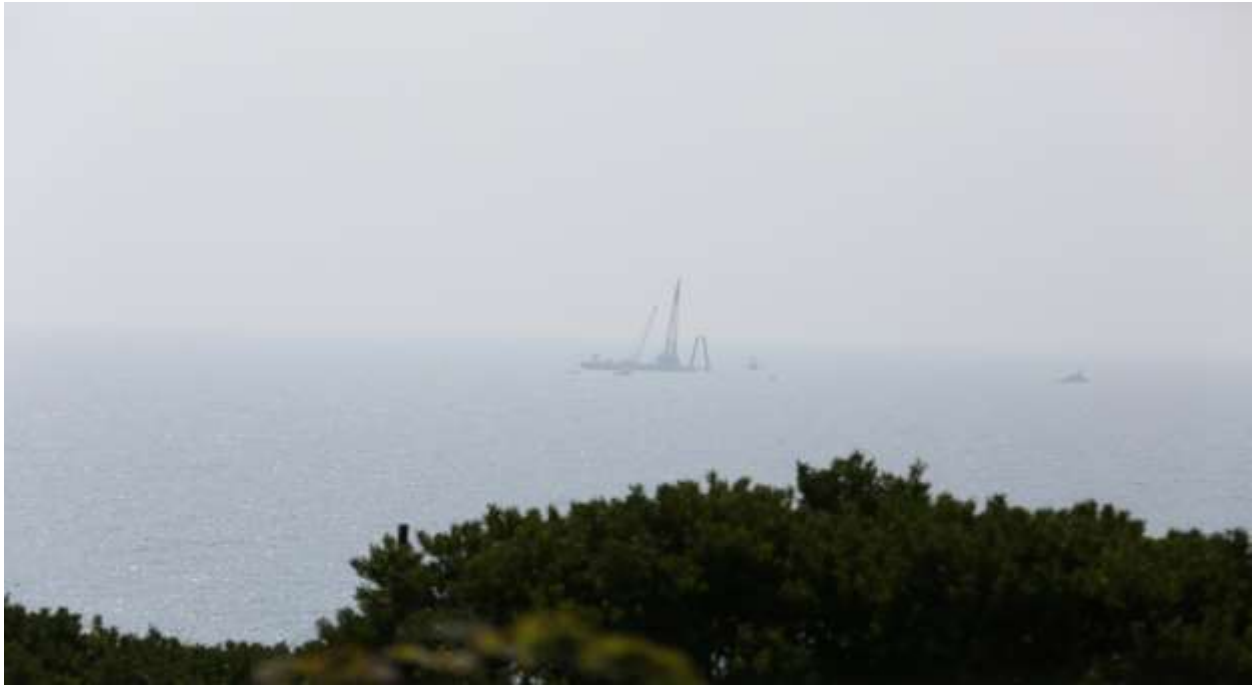
Figure B-4. 08/18/2015 Southeast Lighthouse, Block Island – Photo 0154: Weeks Barge 533 placing the diesel hammer on piling at WTG 2. First day of pile driving.
