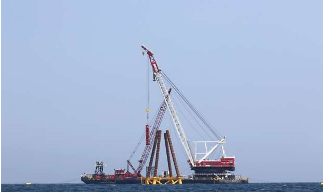
Figure B-7. 08/18/2015 Offshore Photo 0111: Weeks Barge 533 removing diesel hammer from piling at WTG2.
