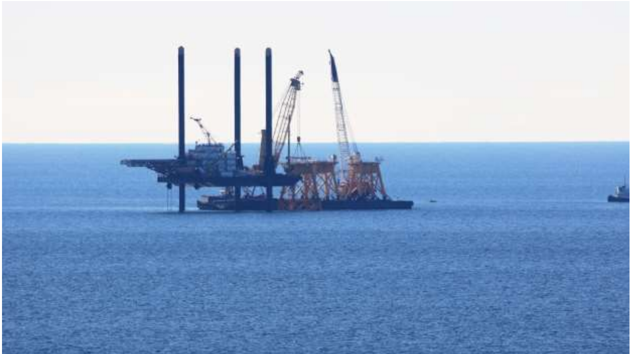
Figure B-18.11/09/2015 Onshore Southeast Lighthouse Photo 2591: Lift Boat Roberts placing transition deck at WTG 4.
