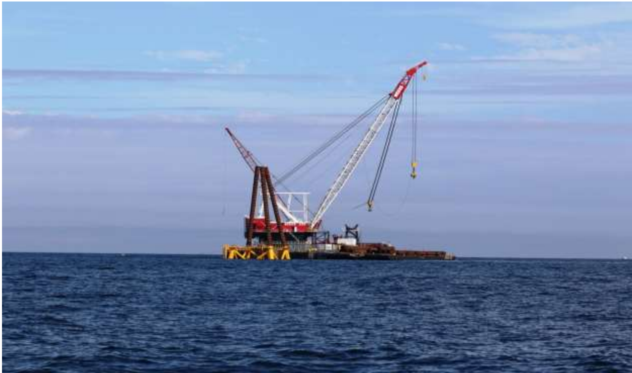
Figure B-10. 8/23/2015 Offshore Photo 0186: Weeks Barge 533 just placed third pile at WTG 3.
