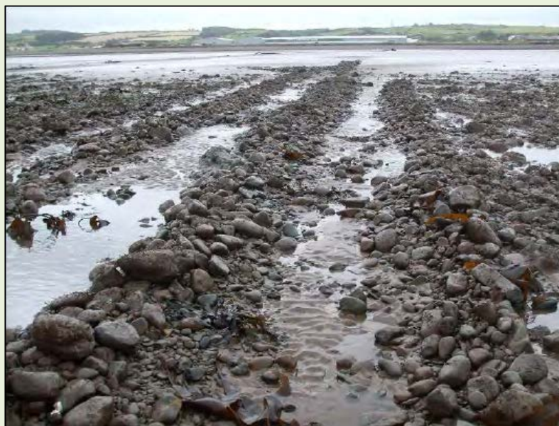
Figure 5.4: Physical impacts of export cable installation on the lower shore at Robin Rigg Offshore Wind Farm (source: Entec, 2009b)
