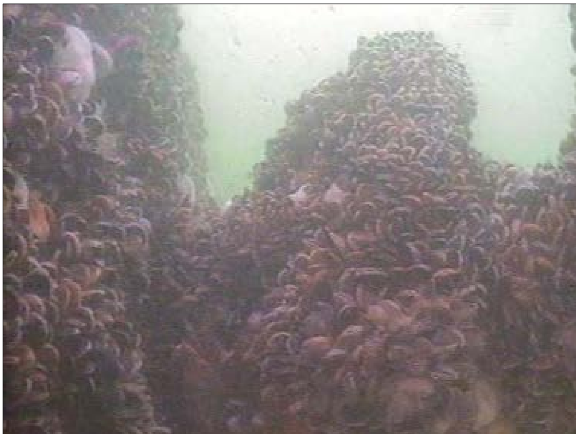
Figure 5.1: Dense mussels ( Mytilus edulis ) with Plumose anemone ( Metridium senile ) attached to a turbine foundation at the Barrow Offshore Wind Farm
