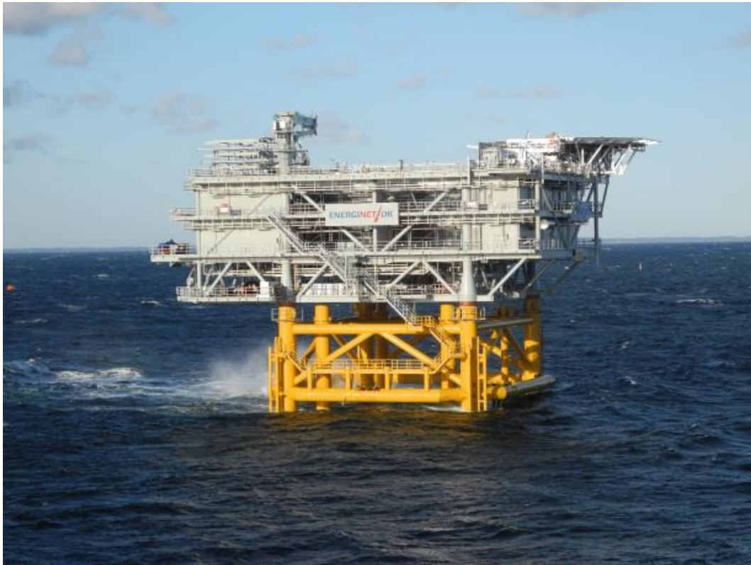
Figure 9: HVAC Offshore platforms at Anholt Offshore Wind Farm (400 MW) (photo Energinet.dk).
