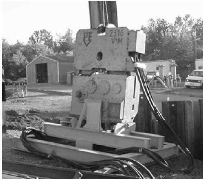
Fig. 8: The PVE 2316 VM driver used for vibratory pile driving (from: Nedwell et al. 2003b).
