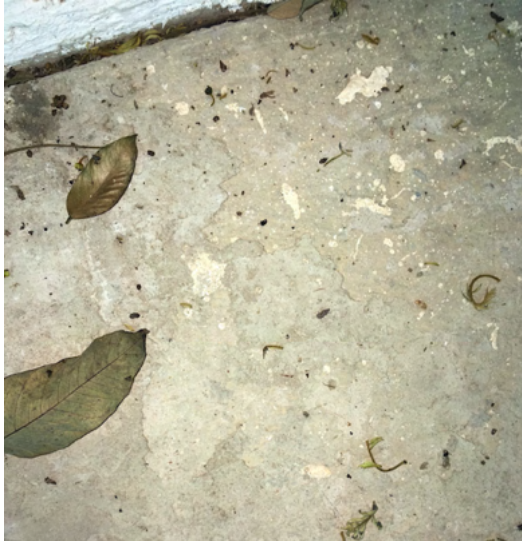
Figure 11: Bat droppings occur at the buildings surrounding the farmhouse, indicating bat presence.
