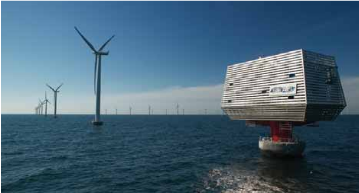
FIGURE 9.5 Transformer station at the Nysted Offshore Wind Farm.
