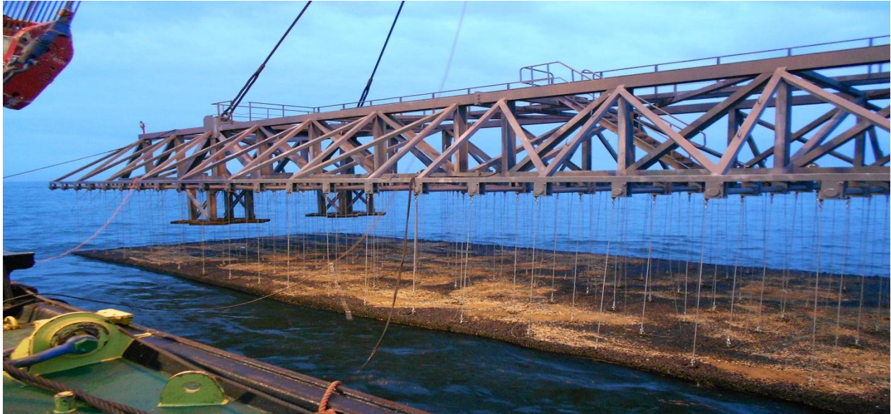
Figure 2: mattresses installation at the Concerto telecom cable crossing (infield cables between area A and B)
