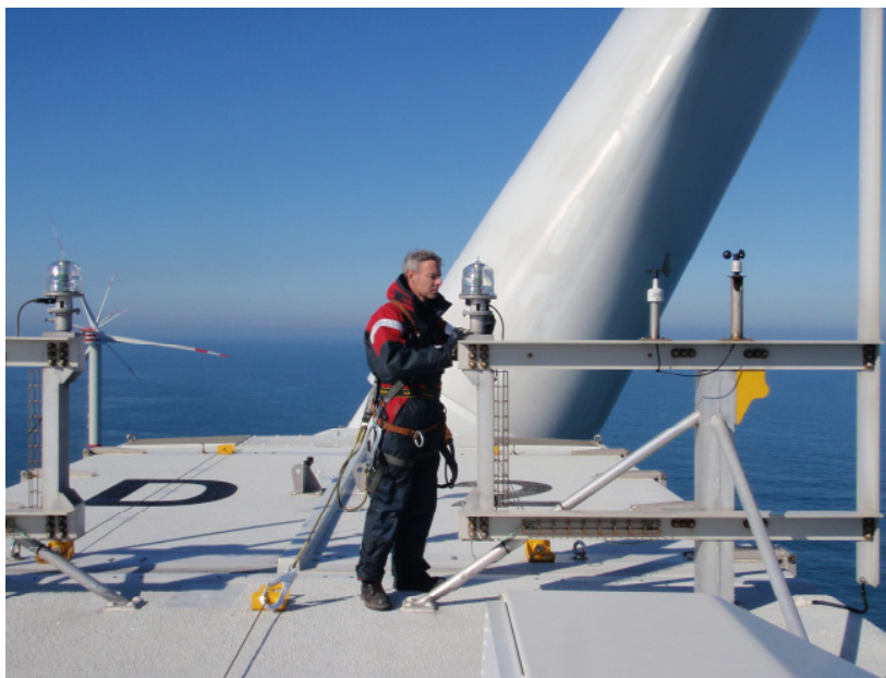
Figure 6 Operational Manager of C-Power safely attached while performing a standard check of the aviation light
