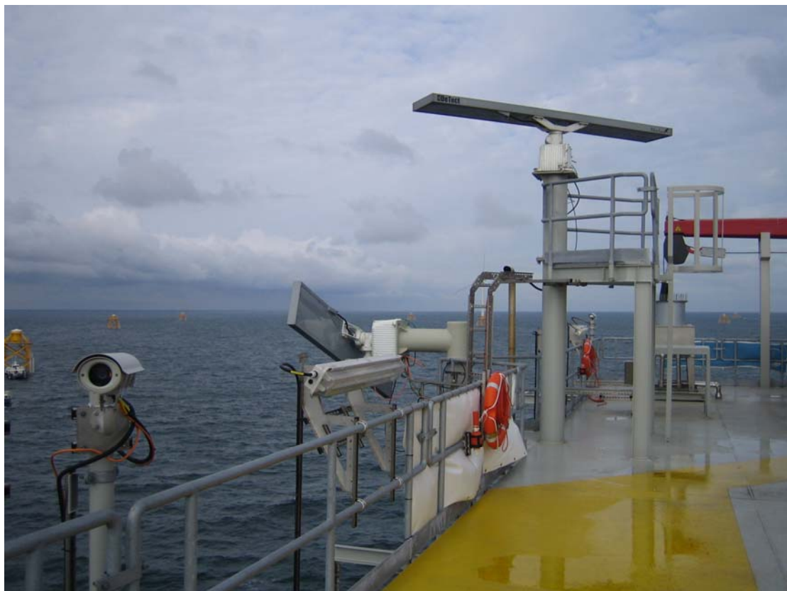
Dual radar system installed on the top deck of the C-Power offshore transformation platform on the Thorntonbank
