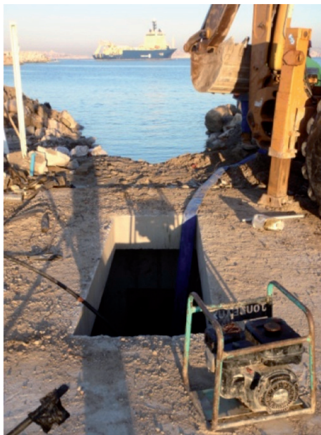
Figure 12. BMH for a telecommunications cable entry in Marseille (France).
