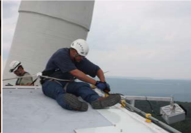
Attaching devices to a safety rail on the top of the turbine nacelle (M. Baker, Bat Conservation International).
