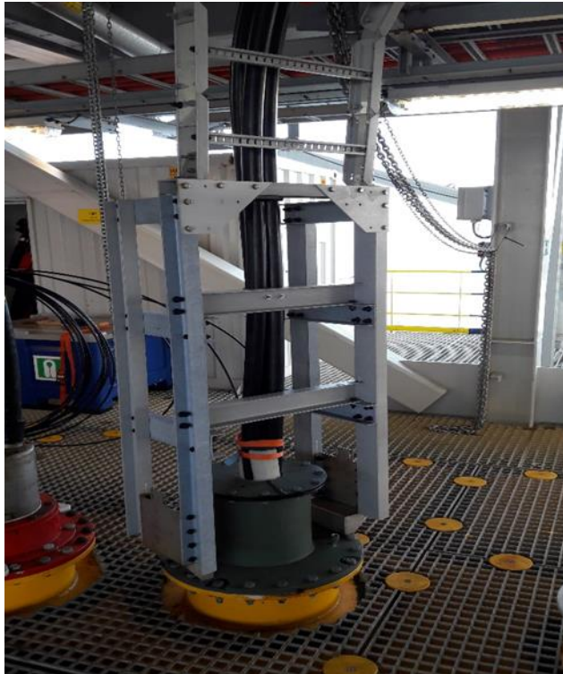
Figure 9: Coupling cable on Belwind OHVS
