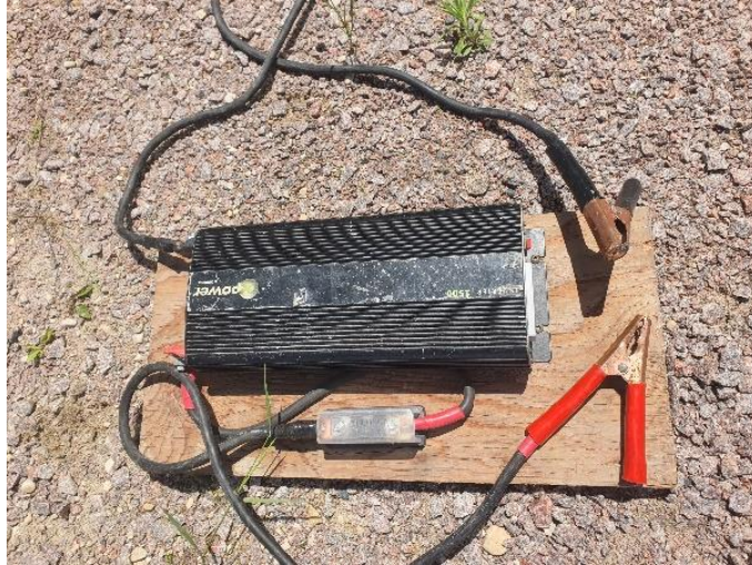
Figure 15: Inverter used to convert 12 V power to 120 V used by laptop, ADCP and ADV instruments
