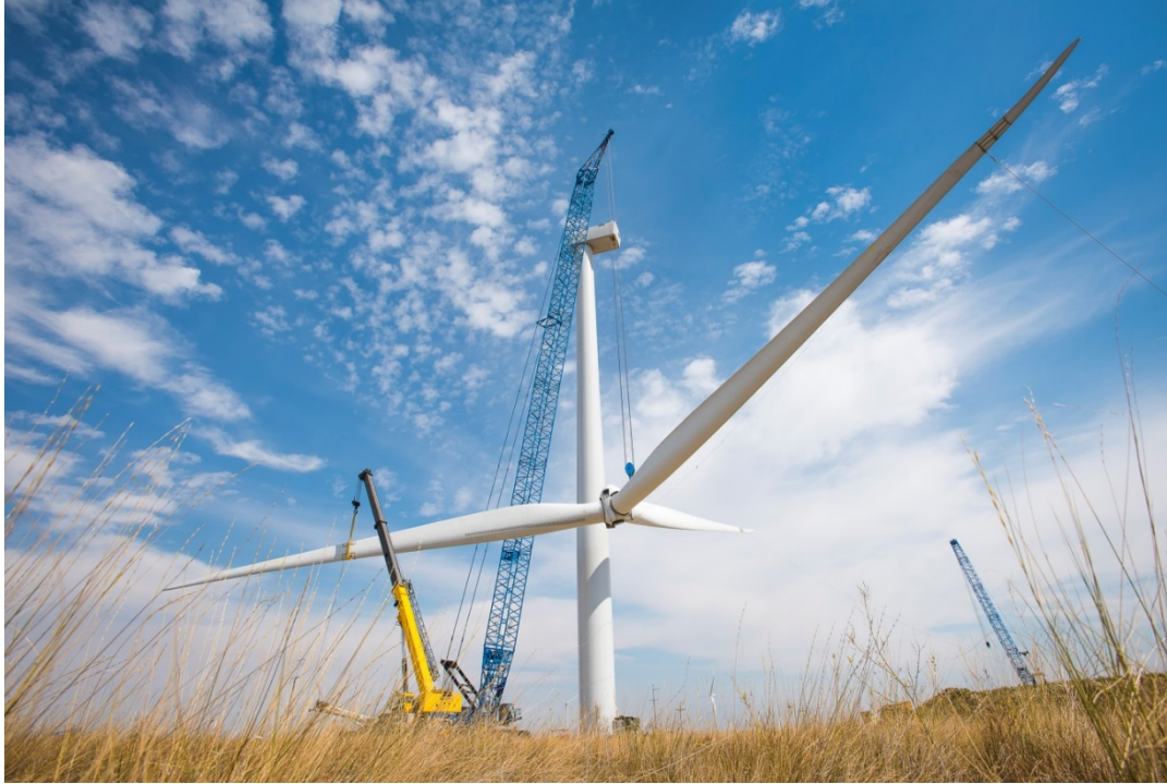
Figure 17. Greenfield Wind, a 25-MW facility located near Fairfield, Montana, was commissioned in September 2016. Photo from Dick Anderson Construction
